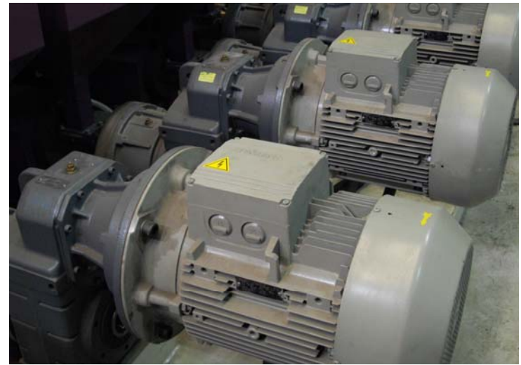
Germany Flender gear box & motor
